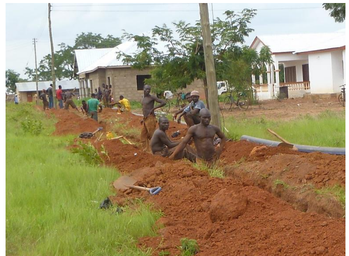
When ditches are dug in Ghana it is almost always done by hand. Fortunately, this ditch means that water is now within a few feet of the new Tamale Institute school building. God is blessing our efforts!
