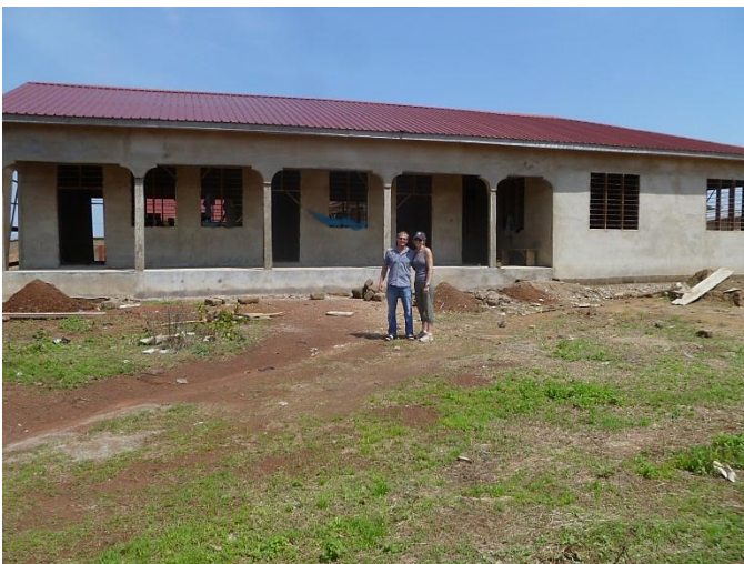
The building project in Tamale is approaching completion as my wife and I pose for the camera. The building has been plastered, windows and doors are being installed, and electricity and water are being hooked up.
