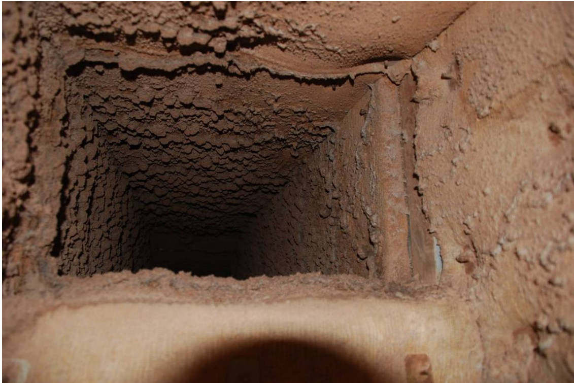
Figure 3 Ducting prior to HVAC hygiene & mould remediation
