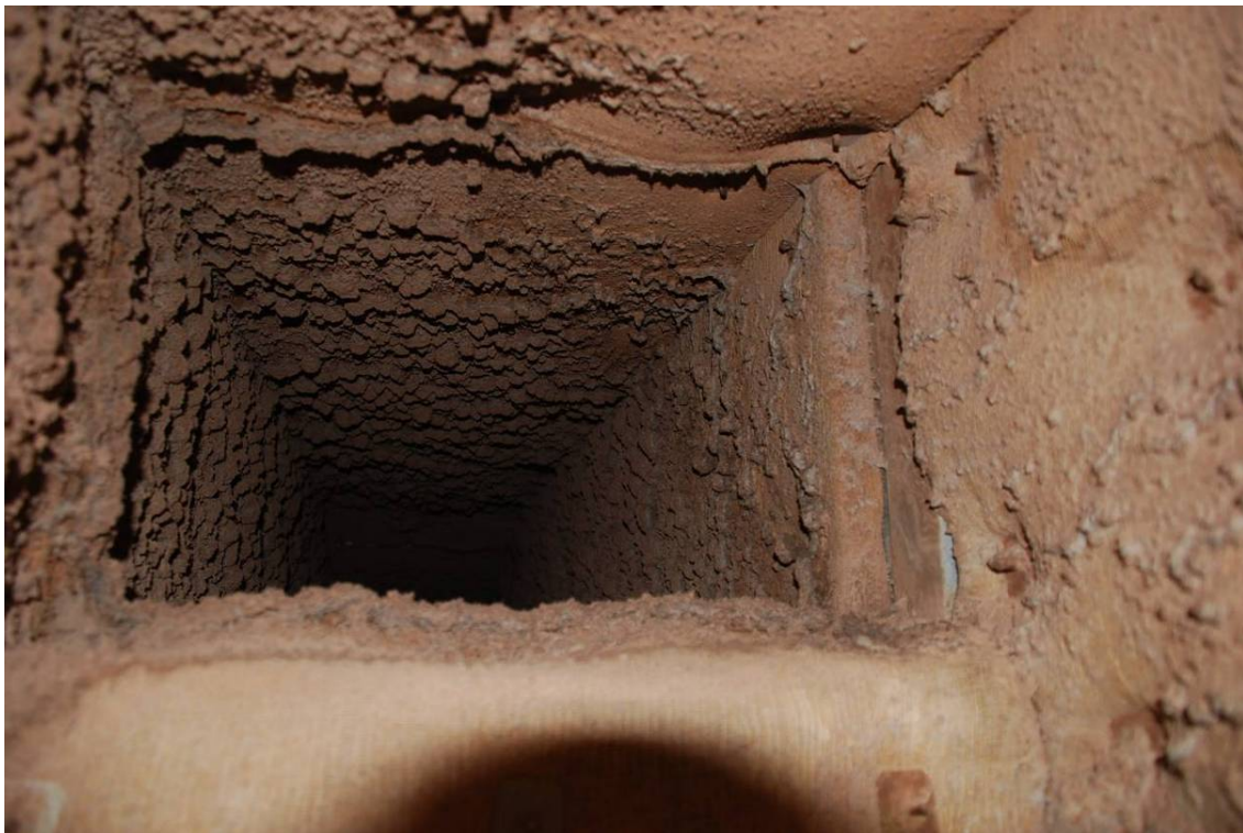
Figure 3 Ducting prior to HVAC hygiene & mould remediation
