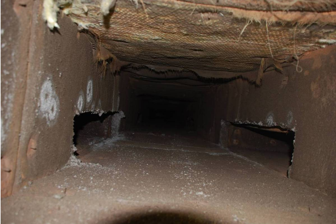
Figure 4 Ducting prior to HVAC hygiene & mould remediation
