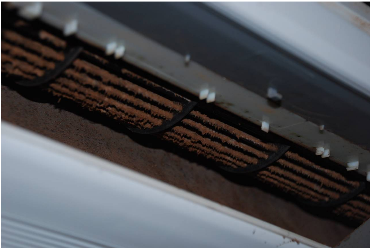
Figure 3 Fan blades prior to hygiene & mould cleaning
