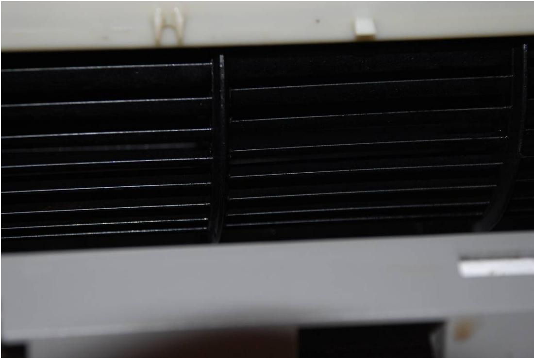
Figure 7 Fan blades after hygiene & mould remediation
