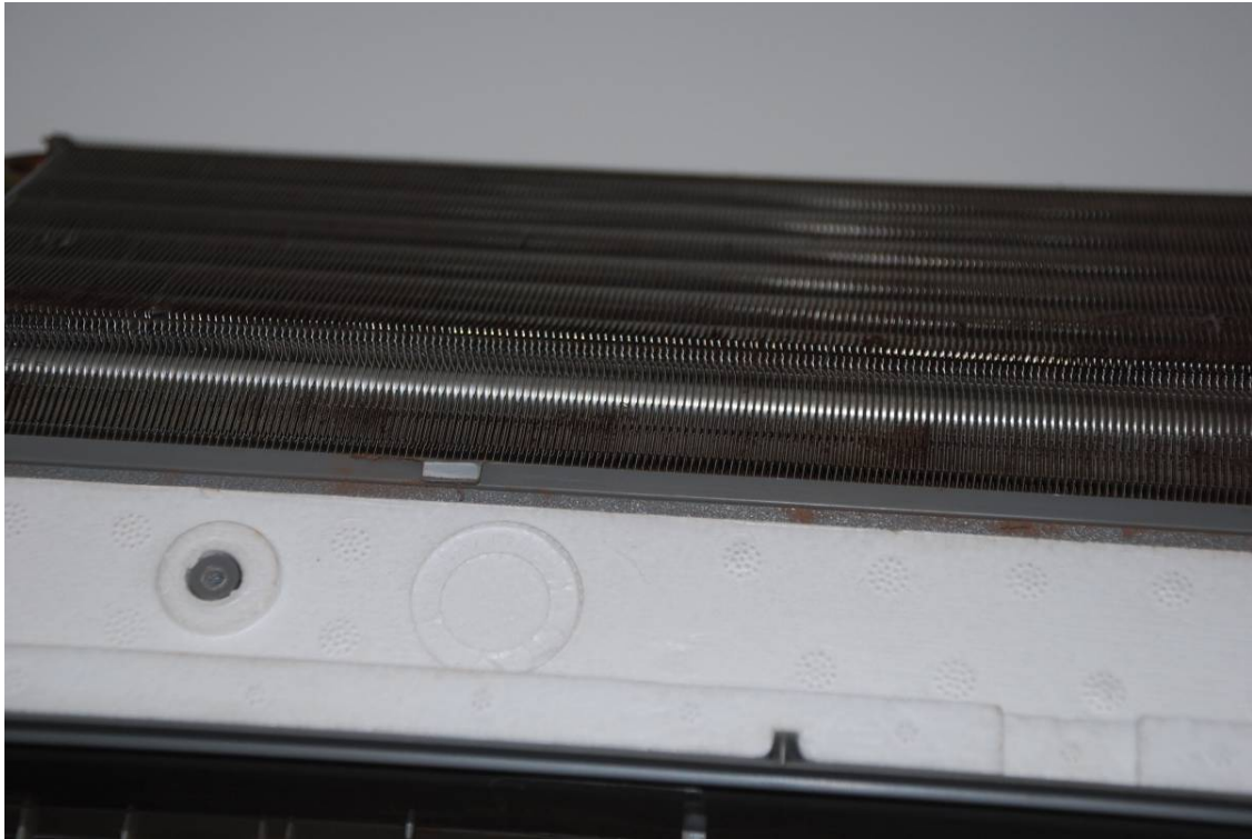
Figure 8 Cooling coils after hygiene & mould cleaning
