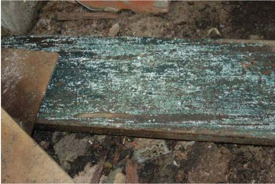
Figure 4 Mould contamination of underside of floor boards
