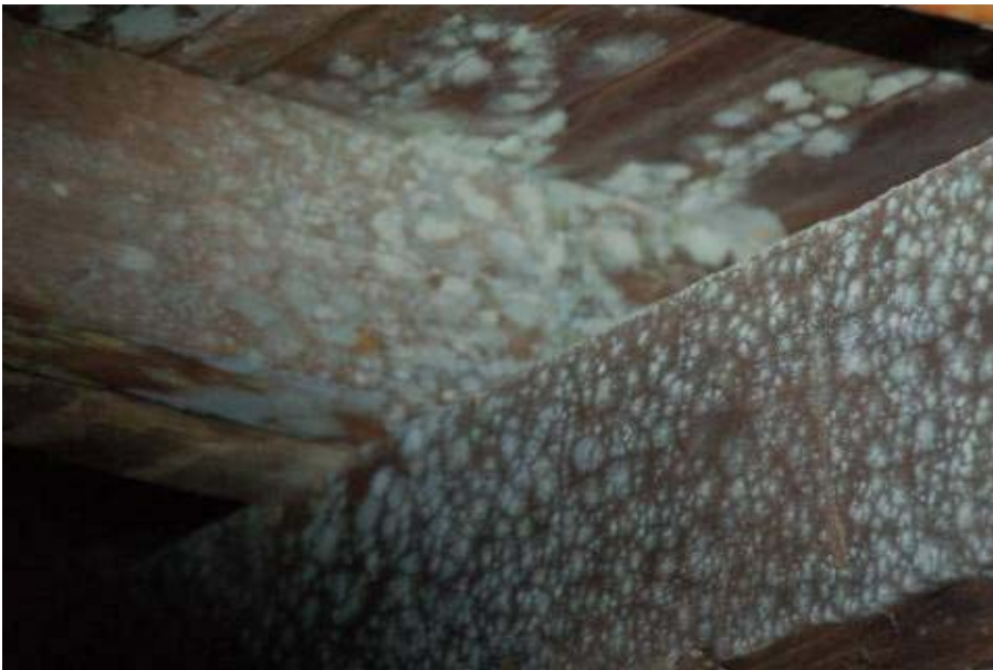
Figure 5 Close up of mould contamination on sub-floor timber
