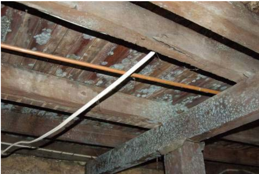
Figure 3 Heavy visible sub-floor mould contamination
