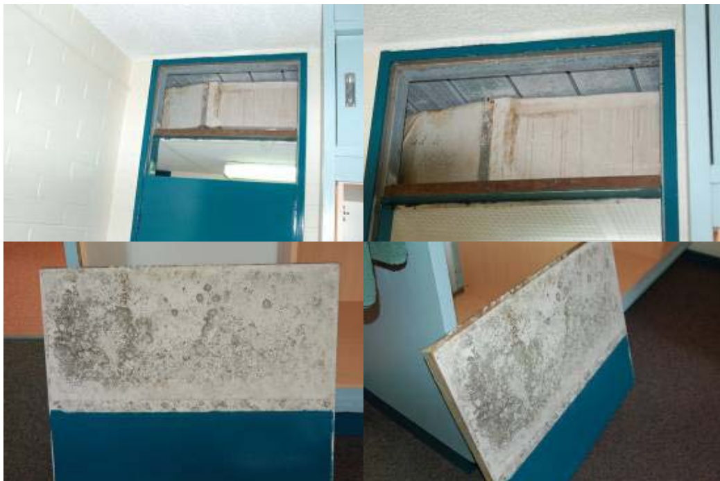
Figure 3 Heavy mould contamination of HVAC ducting and panels
