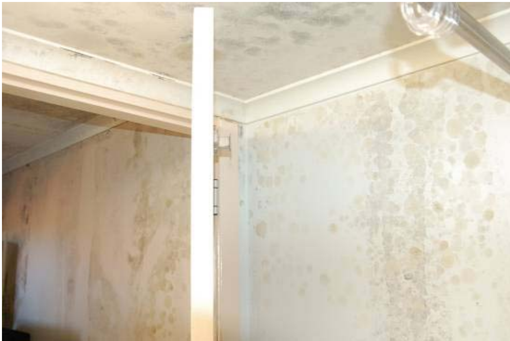
Figure 5 Heavy mould contamination on walls and ceilings
