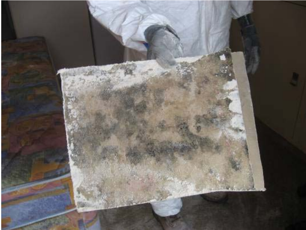
Figure 6 Underside of mould contaminated gyprock ceilings
