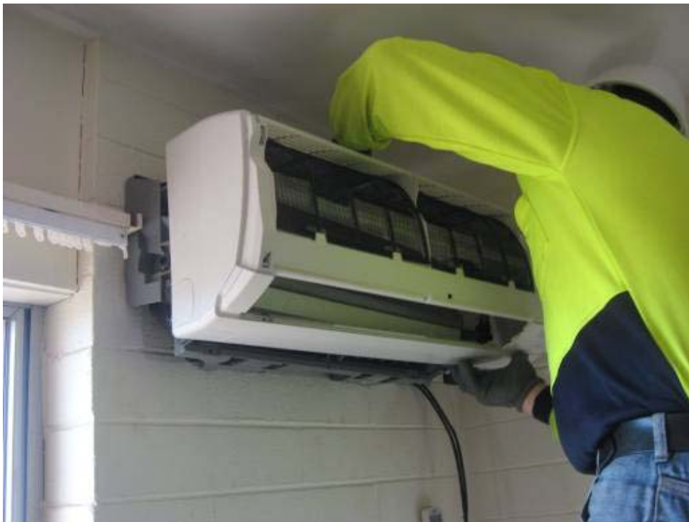
Figure 11 Mould remediation of split system units including coils, fan barrel, fins and filters
