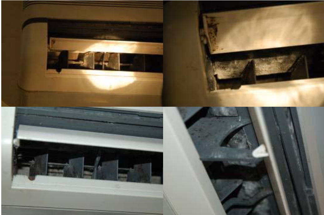
Figure 4 Mould contaminated split air conditioning systems
