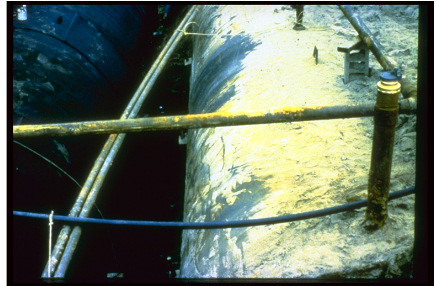
Leaking Underground Fuel Storage Tank
