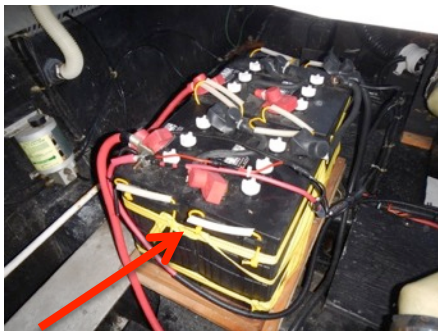
House Bank not secured on plywood sole
