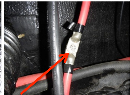
Unprotected positive DC conductors
