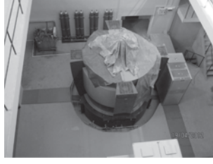
Güneşli HES 1x12,600 MWm 1x12,380 MWe
