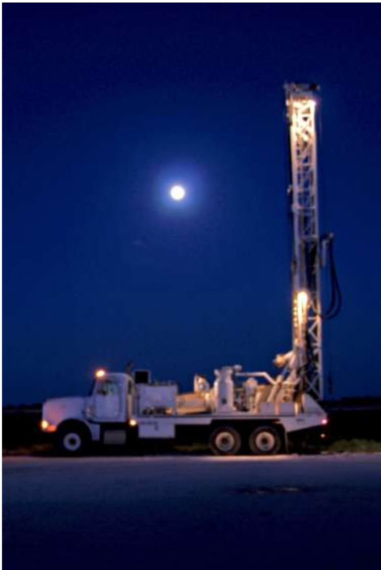
(Straub Corporation photo on the cover of NGWA Water Well Journal October 2008)
