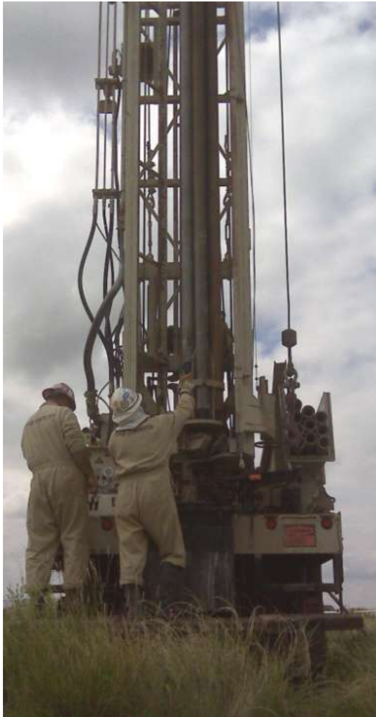
(Straub Corporation photo on the cover of NGWA Water Well Journal August 2010)
