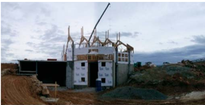
Figure 21. Construction of the winery into the hill side. (Photo Courtesy of Barrel Oak Winery)
